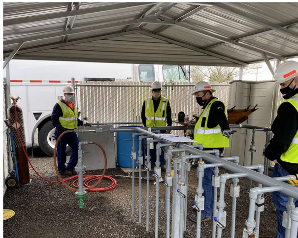
NW Natural employees (left to right) Clay Studtman, Albert Hernandez, Bill Adler and Darin Arnold test hydrogen-blended gas at NW Natural’s Training Town facility.
