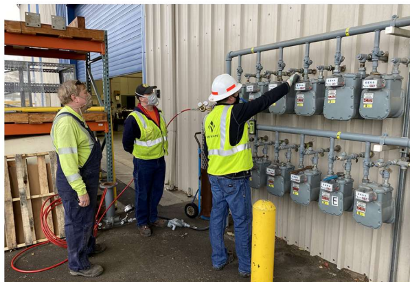
Infrastructure compatibility and leak detection are among the factors that NW Natural and other utilities are testing in their hydrogen blending projects.
